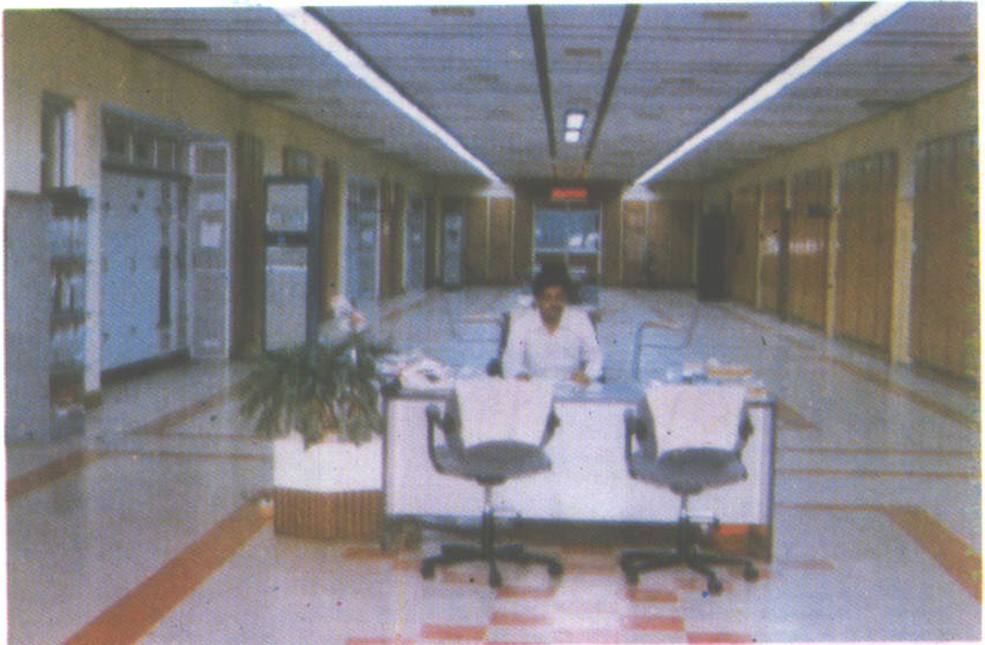
A view of the Transmitter Hall of the 4x500 KW Short Wave Transmitter of All India Radio at Bangalore which is one of the largest of its type in the world.
