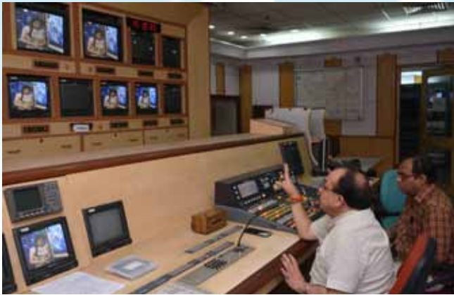
A view of Panel Room at Doordarshan
